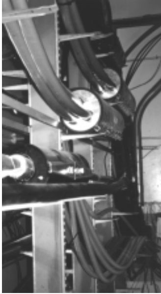
Outside feeder plant enters the CO in the cable vault.
